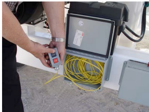
Main Control Panel (Figure1)
